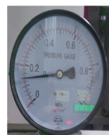
Pressure gauge inside piping
